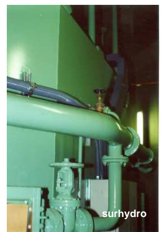
pipe Lines global NAM, SHELL
